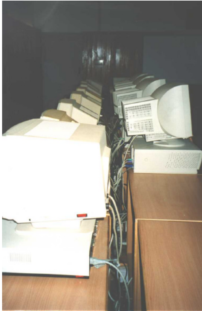
Figure 55: Computer room at Sherubtse College, Kanglung, in the dark as another black-out occurred at the time of visiting the establishment.
